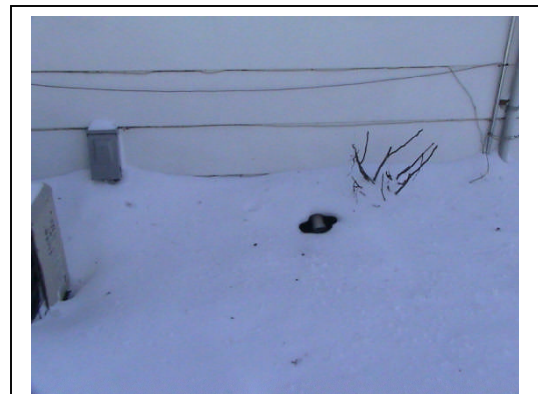
Snow buried flue pipe
