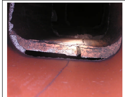
Breached Clay-Tile Chimney Liner
