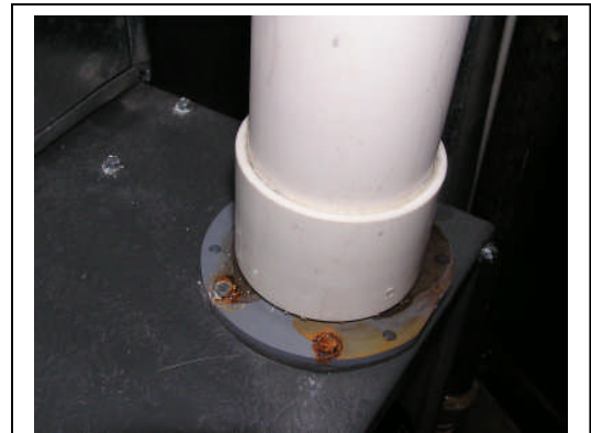
Leaking high-efficiency flue pipe
